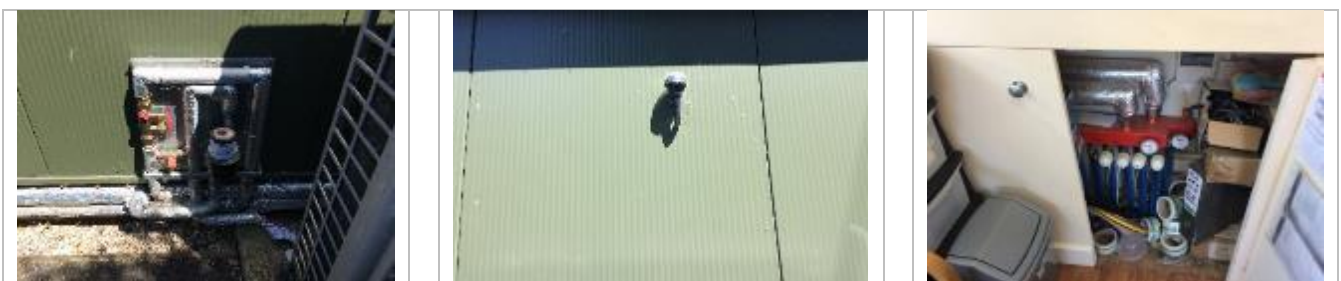
Air sourced heat pump manifold, underfloor heating manifold
