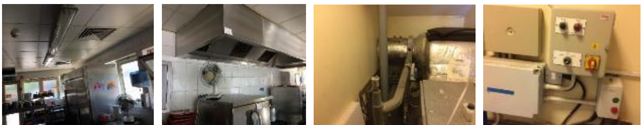
Existing kitchen extract hood and lighting, FA, AHU and controls
