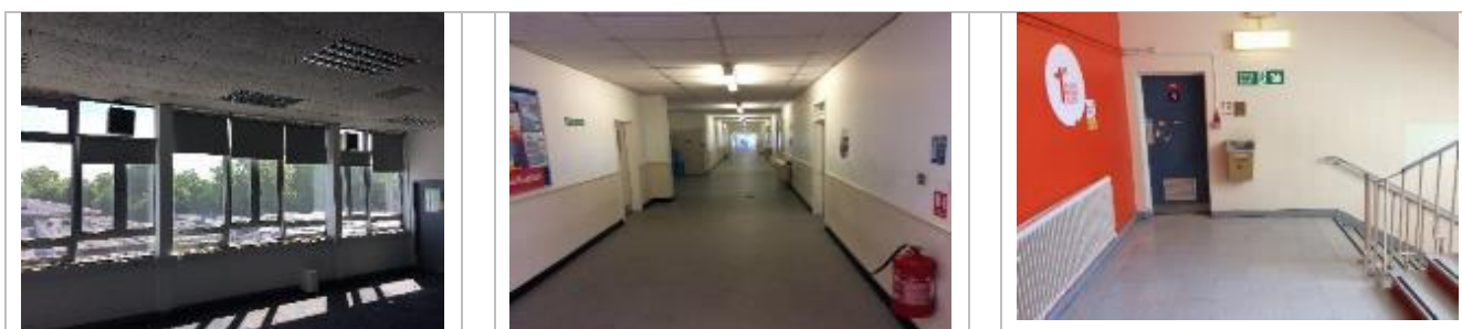
Typical classroom, corridor and stairwell, lighting, htg and FA call points
