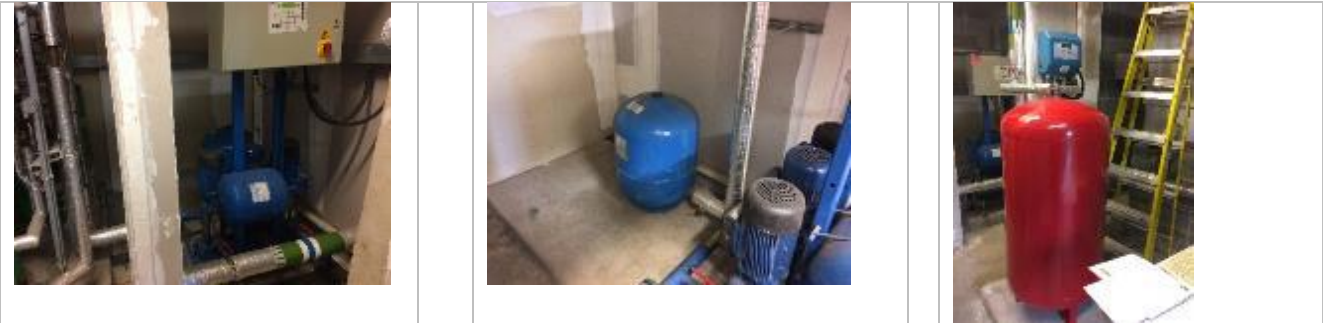
Existing CW Boosters and Expansion Vessels
