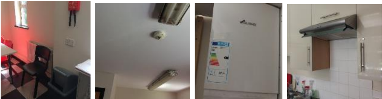
LTHW radiator in kitchenette, FA detection and gas fired boiler, and kitchen extract hood
