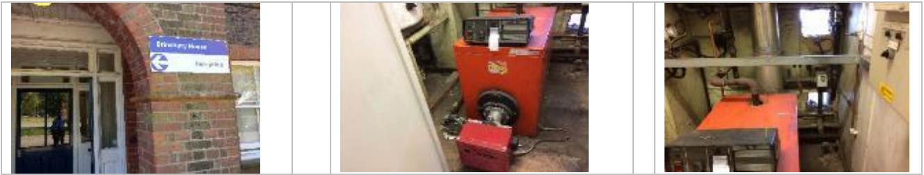
Existing Htg boilers
