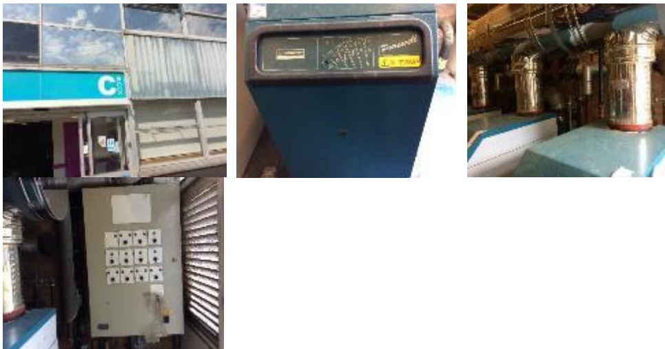
C Block, Existing Boilers and MCCP
