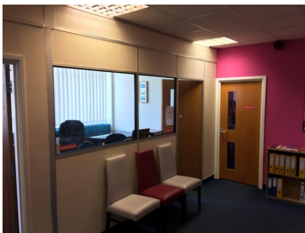
Overview of five internal offices, one with missing smoke head
