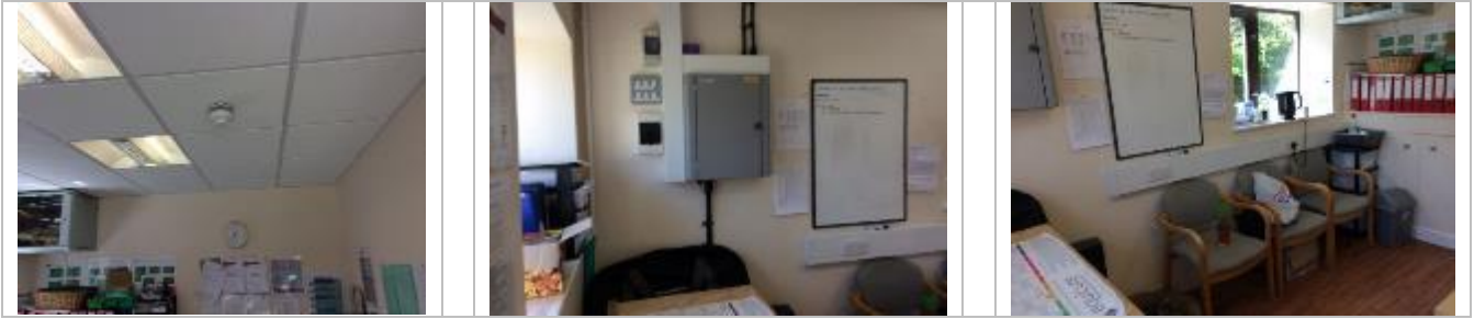
Typical lighting and detector, DB and dado trunking
