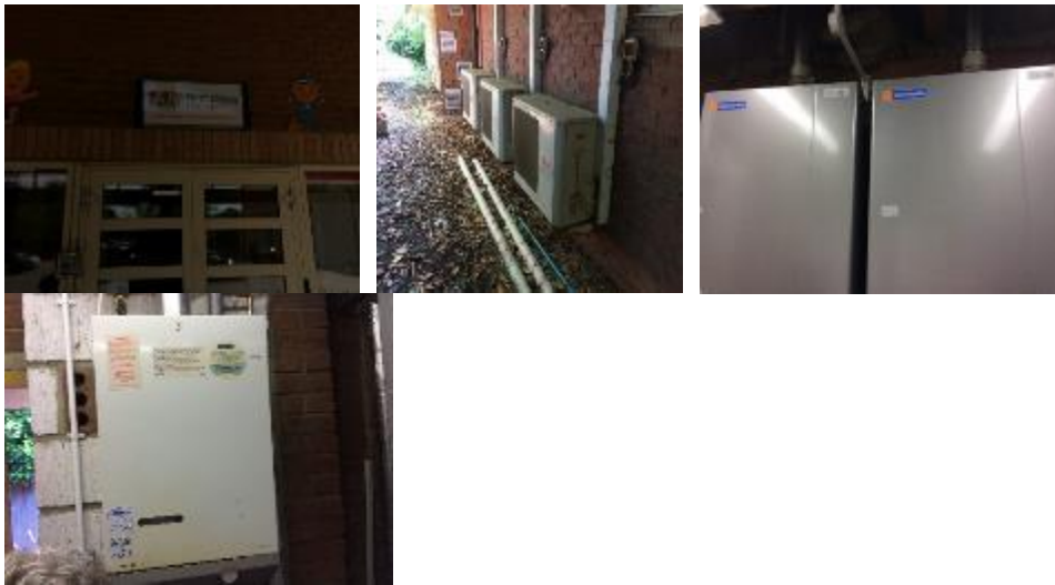
Existing external condenser units, gas fired wall hung Hamworthy boiler providing underfloor heating and Potterton wall hung boiler providing the LTHW to the Megaflo hot water heater.
