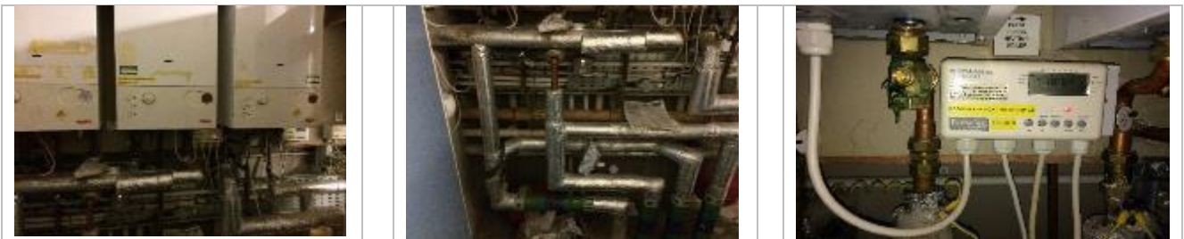
Existing gas fired boiler serving Longley I, Note these are contained within a cupboard. Access is difficult for maintenance and there appears to be no ventilation.
