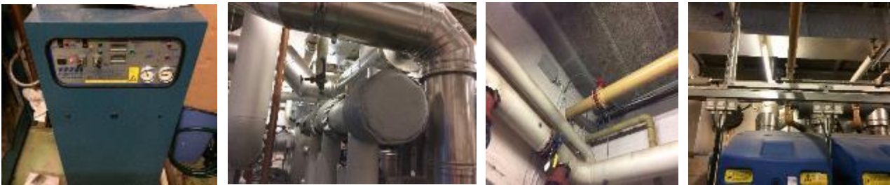
Existing pressurisation unit, flues, automatic gas shut off valve and gas detection over boilers
