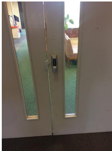
Visible gap between double door set
