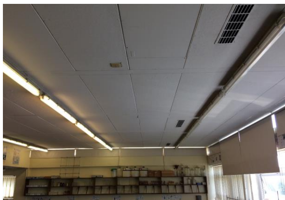
Laboratory with no fire detection
