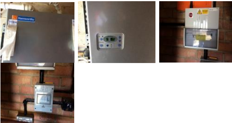
Existing wall hung gas fired LTHW boiler, electrical consumer unit
