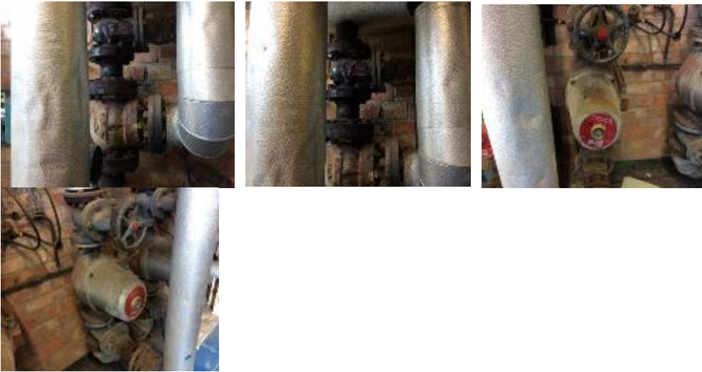
Existing Htg Valves, pipework and pumps within the plantroom. Condition poor
