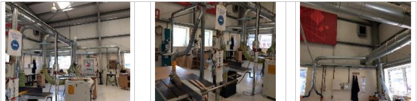
Extract system to equipment & ducting at high level with supply grille at high level
