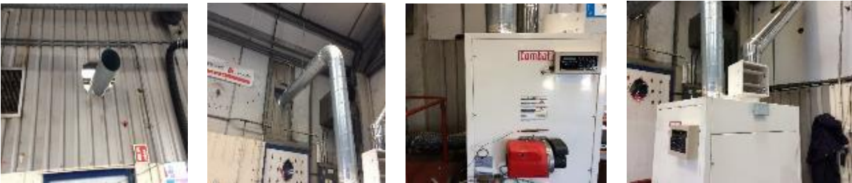
Warm air duct providing heating to workshop, oil-fired warm air heater.
