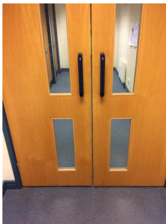
Visible gap between cross corridor door set
