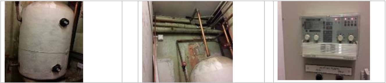
Existing HW cylinder and Htg controls
