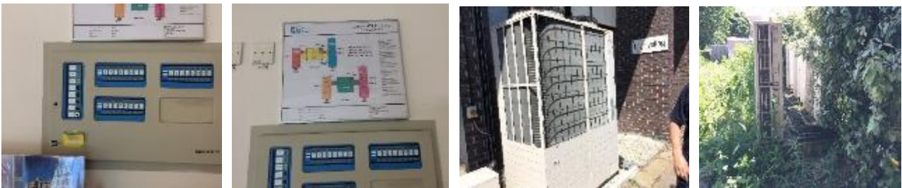
FA panel and zone plane, external air cooled condensers.
