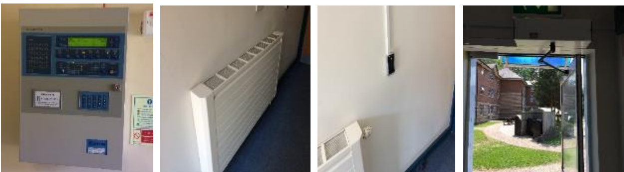
FA panel common to blocks, LSTR and access control with automatic door for disabled.
