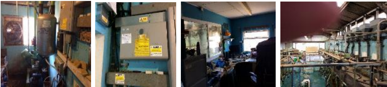
General electrical DB, office and milking parlour
