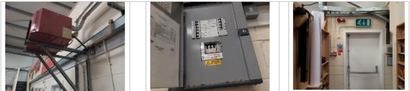
Direct gas fired unit heater, DB and emergency escape route
