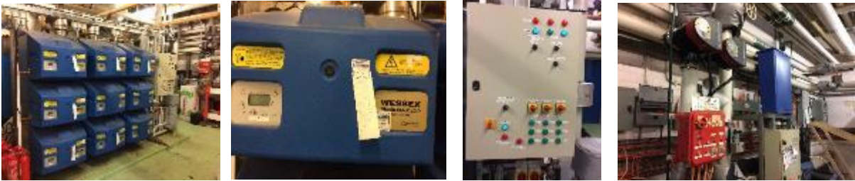
Existing gas fired Modular Boilers, Control panel and zone 3 htg variable speed pumps
