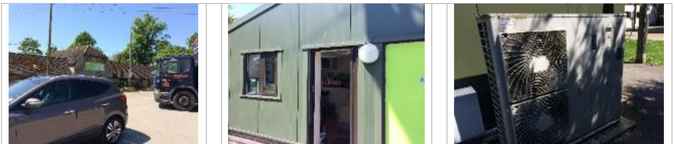
Office and air source heat pump unit
