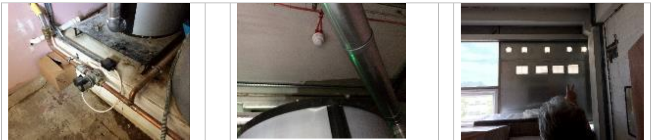
Gas shut off valve, fire detection & ventilation for combustion air.
