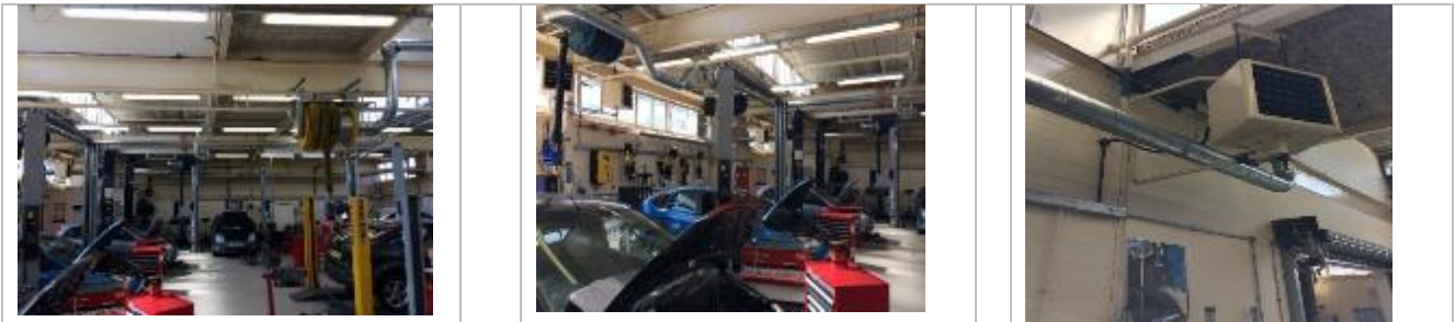
Car maintenance workshop, local extract for exhaust extraction and unit heater
