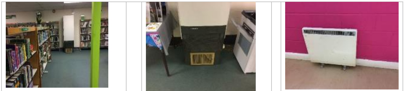
Electric heating units and panel radiator
