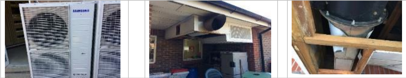
External condensers, kitchen extract and supply unit
