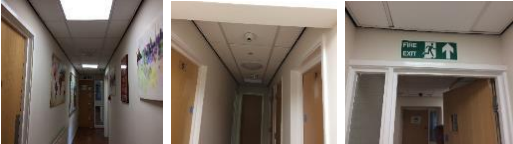
Typical corridor Lighting, FA and Fire detection
