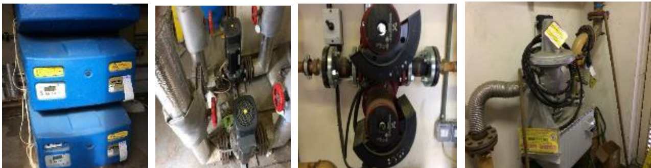
Existing modular boilers, heating pumps and gas meter.
