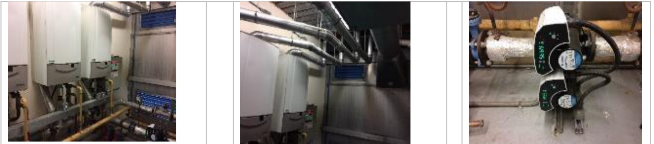
Existing Remeha gas fired boilers, serving Longley II, but located in Longley I & VSD pumps
