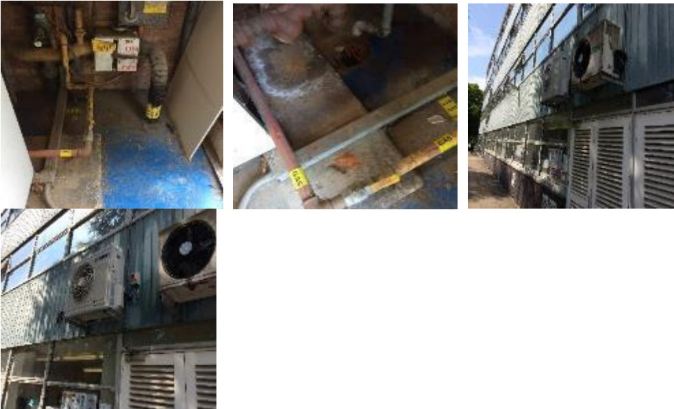
Existing gas incoming main, gas valve and pipework, existing external condensers, one in poor condition.
