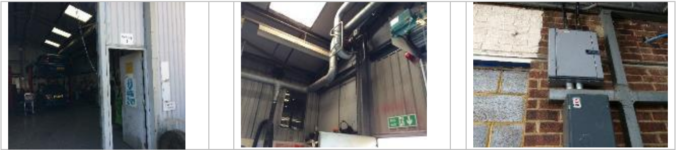
Existing exhaust extract system and DB.
