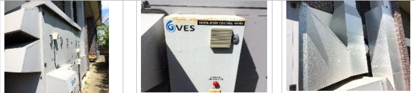
External heat recovery air handling unit
