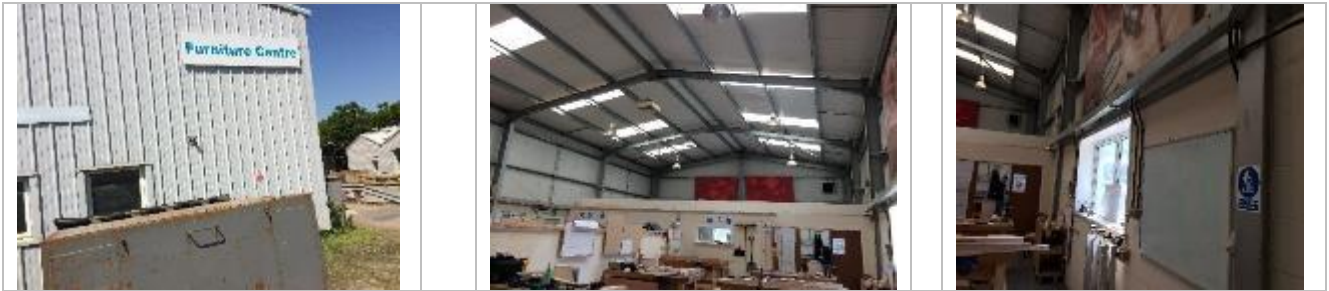
High level lighting, fire detection and electrical containment
