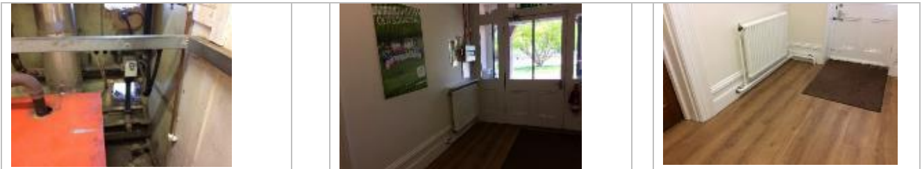
Existing port valve arrangement & radiators
