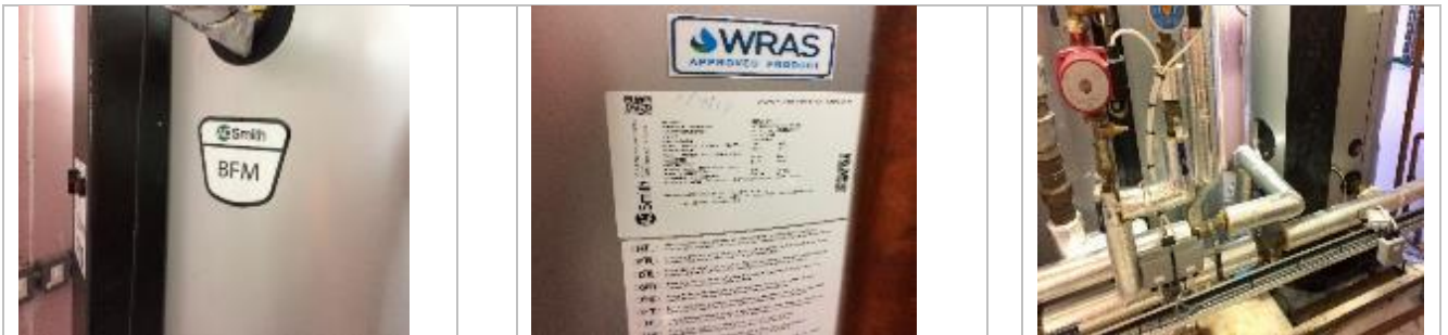
Hot water Gas fired Water Heaters & HWS secondary return pump
