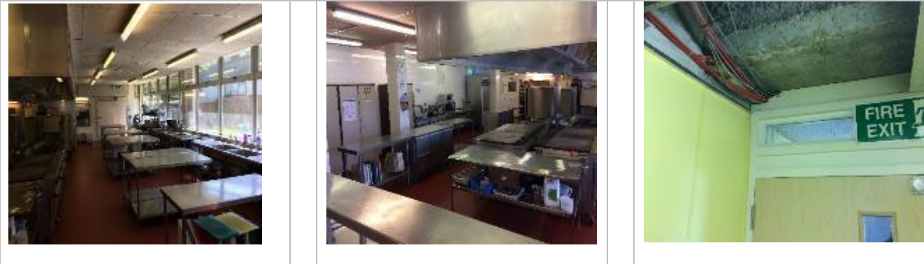
Production kitchen and exposed electrical services requiring attention/making good of compartmentation
