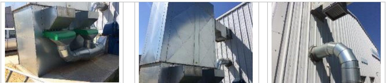
External recycling filter and fan combination unit.
