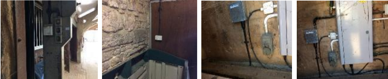
Existing light switches, sockets, and main DB
