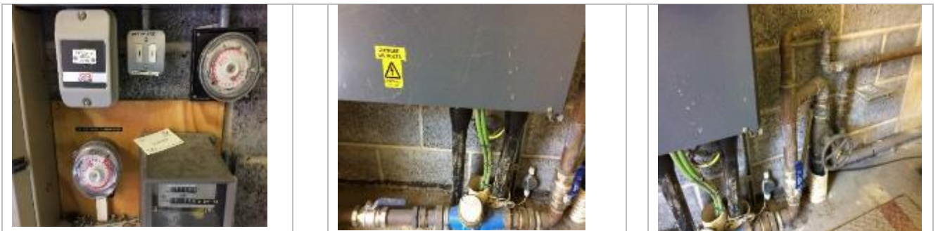
Metering, main electrical incomer and main incoming water main
