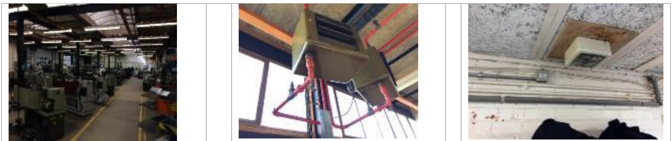
General engineering classrooms, typical unit heater within workshops, local extract unit through roof
