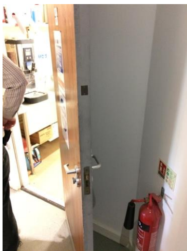
No intumescent strips or smoke seals to the marked fire door between the kitchen and café
