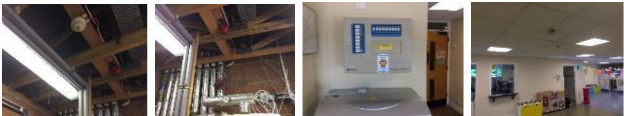
Existing FA heat/smoke and sounder, security system and classroom fire heat/smoke detector.
