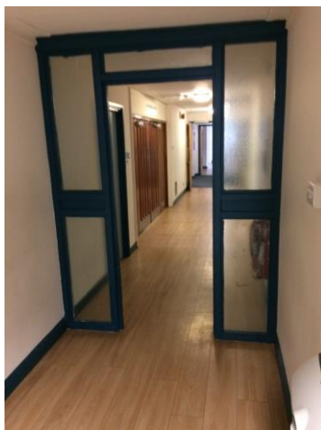
Cross corridor door set absent
