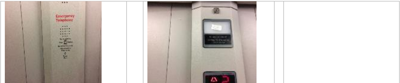
Existing lift in central atrium serving both blocks
