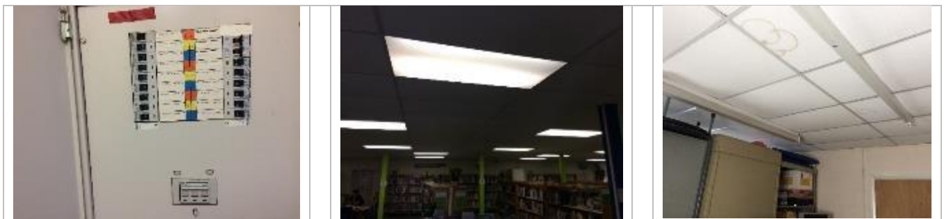
General DB and typical lighting
