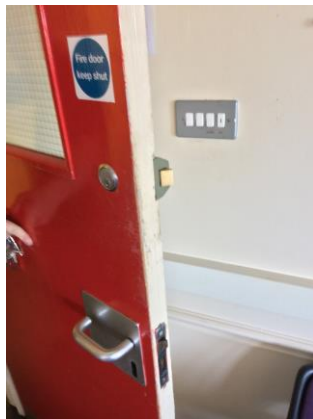
No intumescent strip or smoke seal to door marked as fire door
