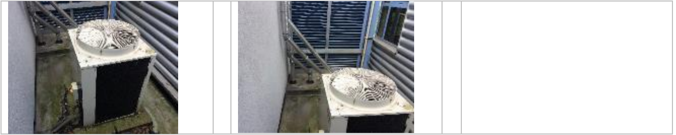
Existing Condenser at mezzanine roof level
