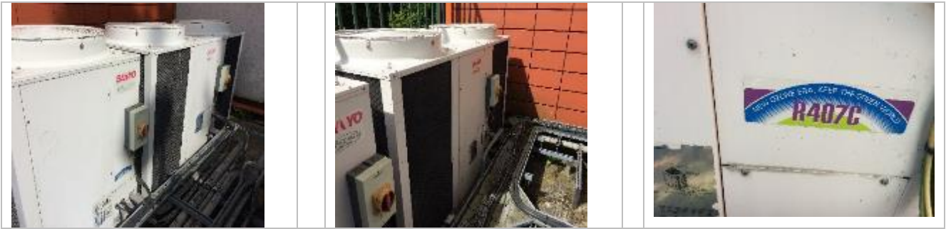
Existing Multi-splits condenser units serving Longley II
