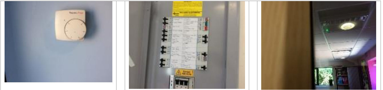
Underfloor heating room sensor, DB and classroom emergency light fitting
