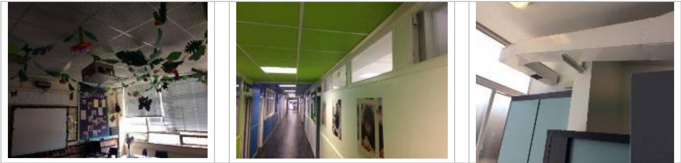
Typical classroom, corridor and toilet extract.
