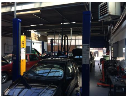
No fire detection within motor vehicle workshop
