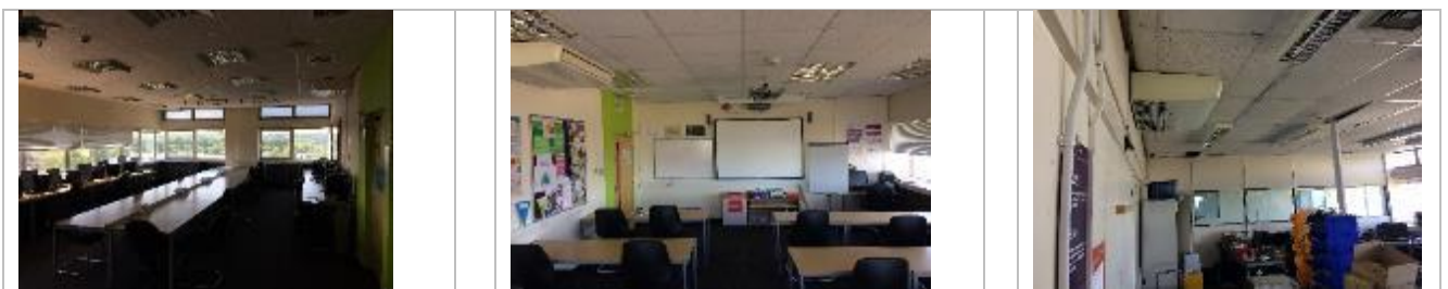
Typical tower classroom dado trunking for small power, split AC unit and perimeter Htg
