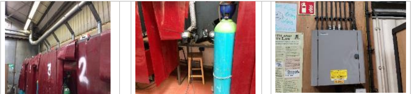
Welding booth extract system & electrical DB
