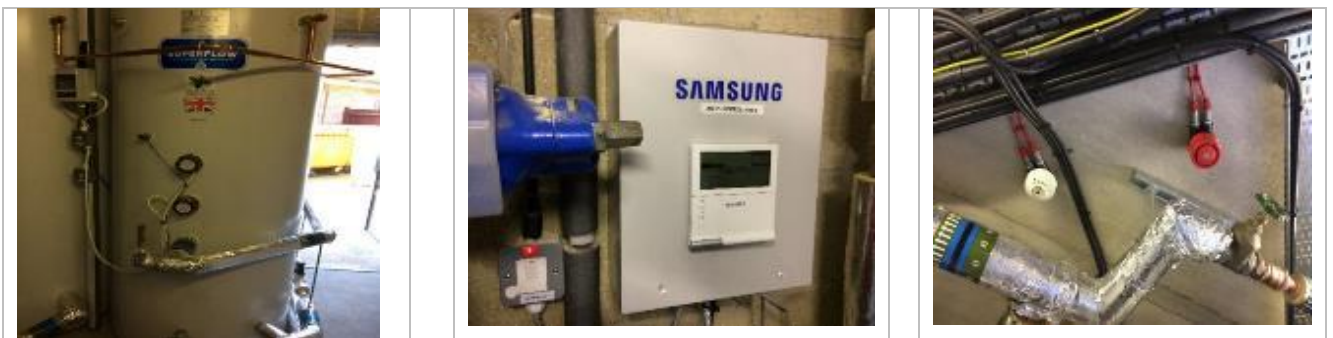
Hot water cylinder, ASHP control and fire detection within plant room
