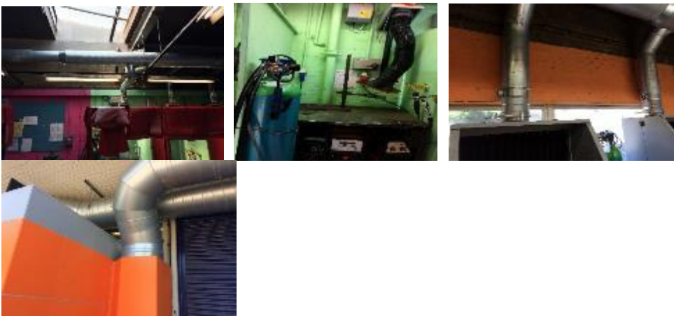
Welding booth extract, forge extract and recirculation ventilation unit.
