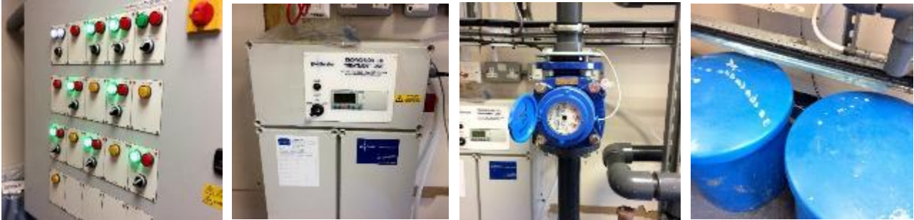
MCCP, Legionella treatment plant
