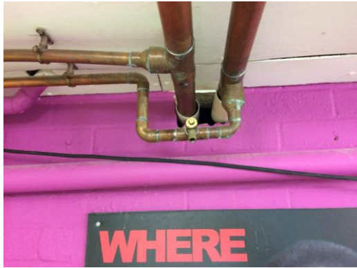
Service penetrations through common room solid walls
