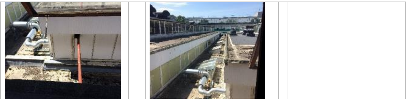
Existing roof mounted extract fans from workshops
