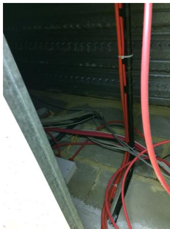
Fire compartmentation breach due to service penetrations
