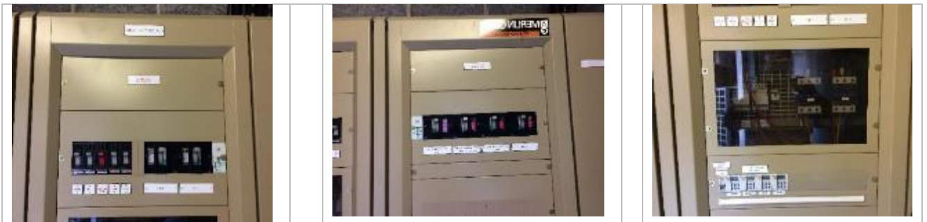
Main switch panel
