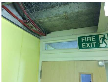
Fire compartmentation breach due to service penetrations
