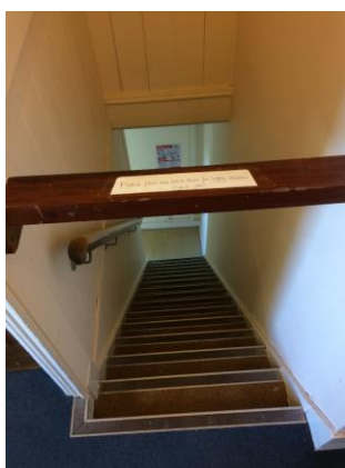
Secondary staircase which may not be suitable as a means of escape (if designated)
