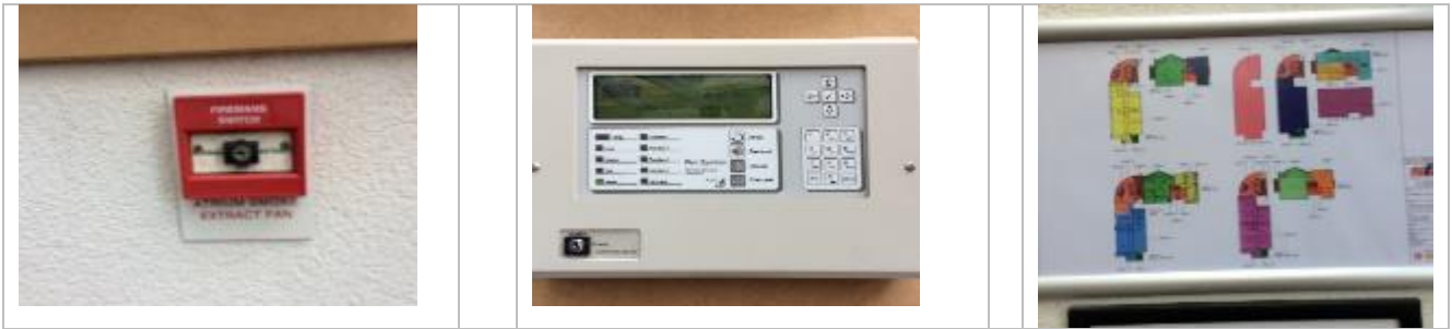
Fire safety system and atrium smoke fan control.
