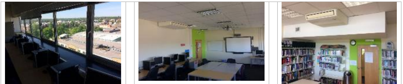
Typical tower classroom dado trunking for small power, split AC unit and perimeter Htg
