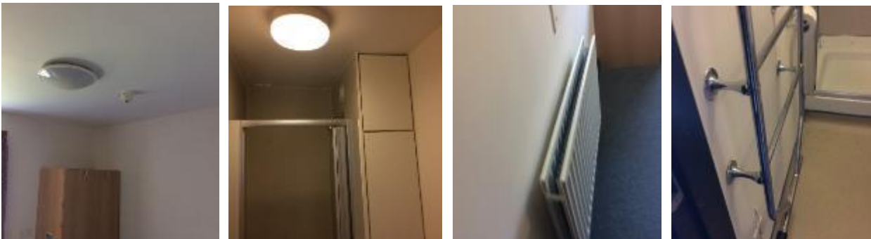
Student flat, FA detection, toilet extract (central system) LTHW radiator with TRV and electric heated towel rail.
