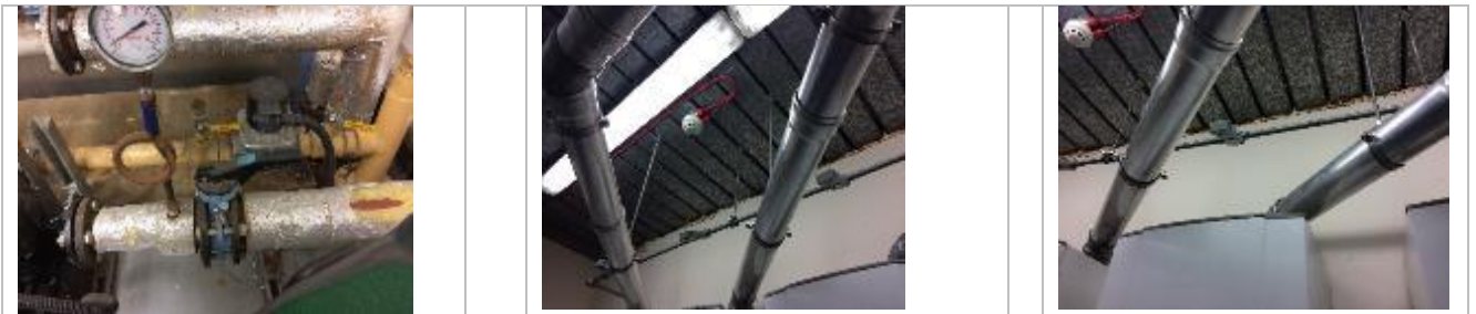
Gas solenoid valve, gas detection and heat/smoke detection
