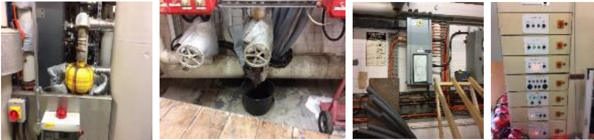
Plant and valve leaking, DB and MCCP.
