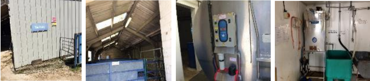
Dairy pasteurisation vessel and storage
